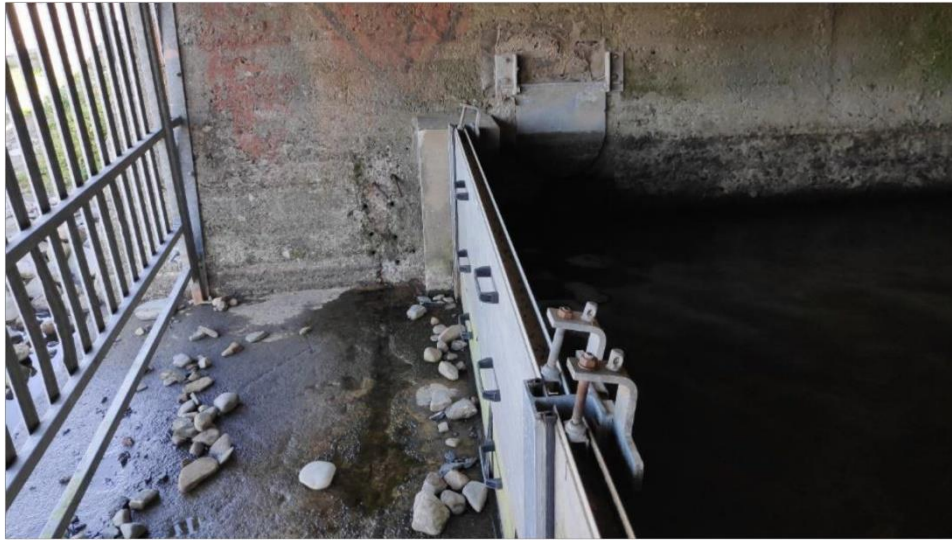
Plate 3.9 The tidal gate at the sea outfall of the Kilkee Upper Stream (under the Marine Parade Road) is a barrier to eel passage during summer. The barrier is opened after the bathing season (4 th June to 31 st August)
