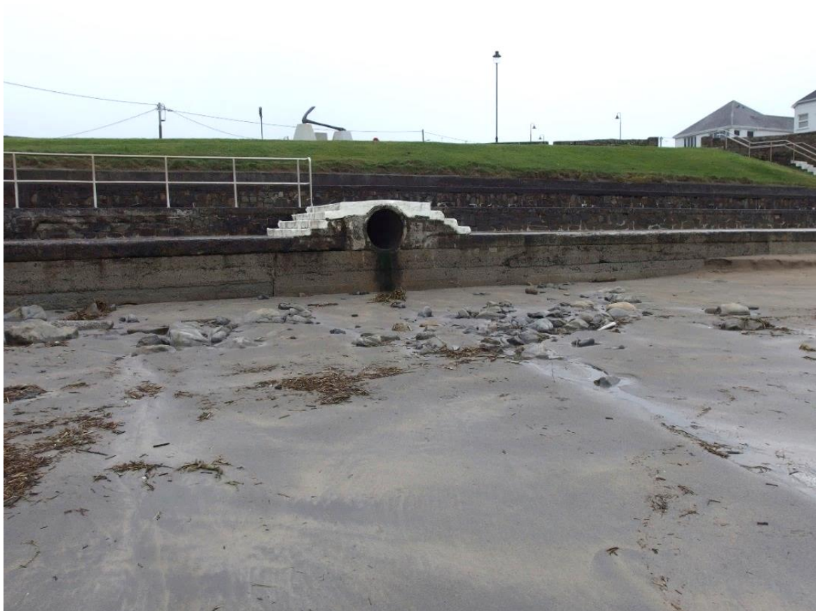
Figure 7-11: Atlantic Stream culvert overflow
