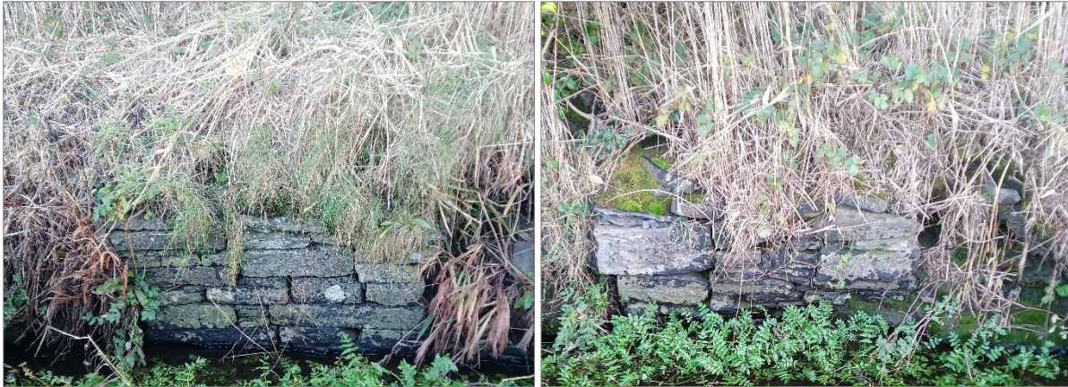
Figure 11-16: Drystone wall sections along the south bank in Area 1 taken from the northwest.
