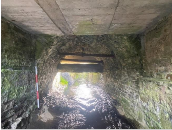
Transition between north-western extension and original stone bridge face taken from the northwest.
