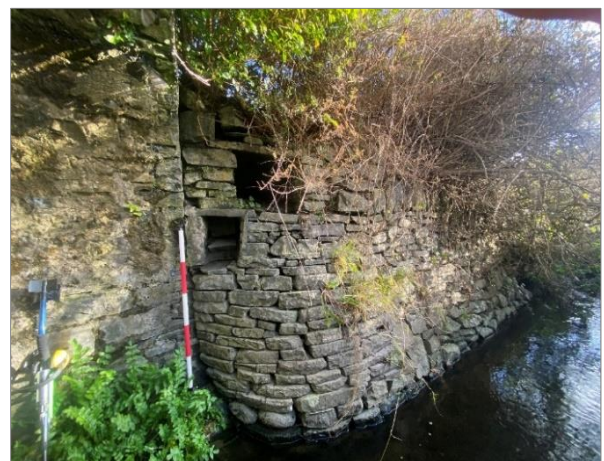
Northeast stone revetment wall with two drains seen when viewed from the southwest and varied construction periods evident.
