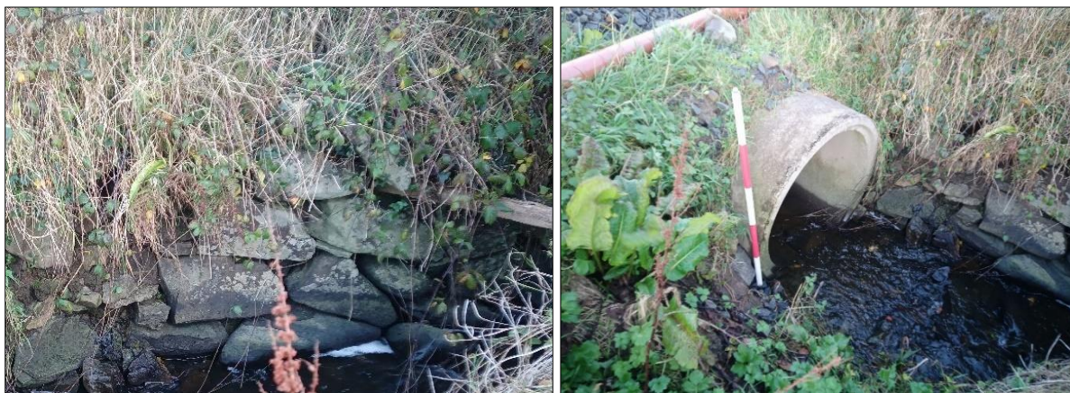
Figure 11-15: Drystone boulder wall in Area 8. Left: taken from the west-southwest. Right: with concrete culvert taken from the south-southwest.
