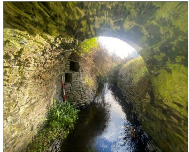
View of stream entering the bridge with drystone wall on either bank taken from the northwest. Various phase of construction is evident within the bridge structure, including the earliest phases.
