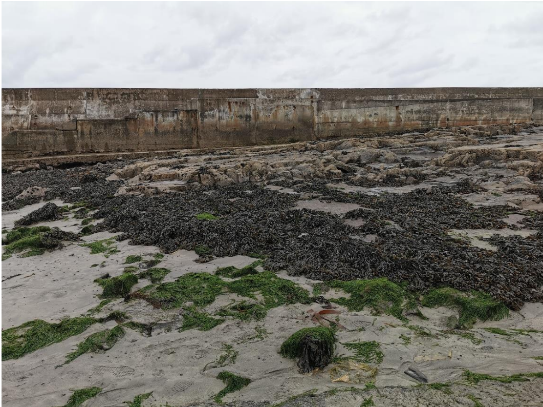
Figure 5-7: Rocky shore behind sea wall with seaweed growth on rocks, intact bedrock with rock pools.
