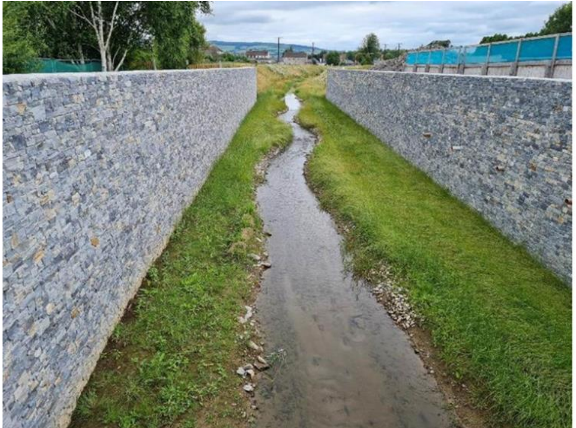
Figure 8-2: Sample Visualisation of the new U-channel within the flood walls (Image for illustration purpose from Templemore FRS – (Tobin 2022)).
