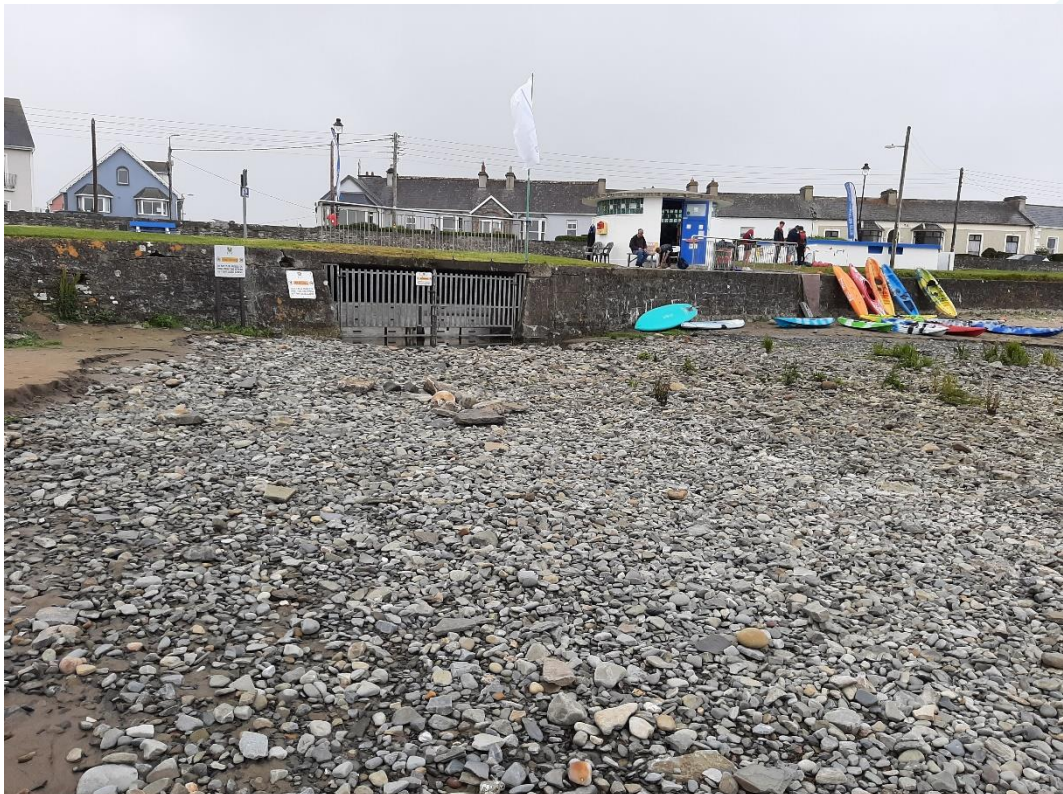
Figure: 5-3 Victoria Stream culvert main outfall with stop log and gate in place.
