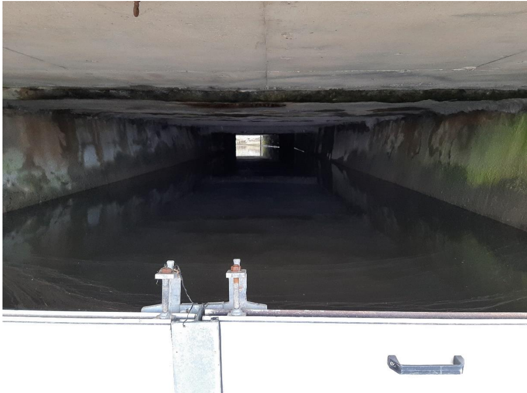
Figure 5-4: Victoria Stream culvert main outfall with stop log in place looking upstream through box culvert.
